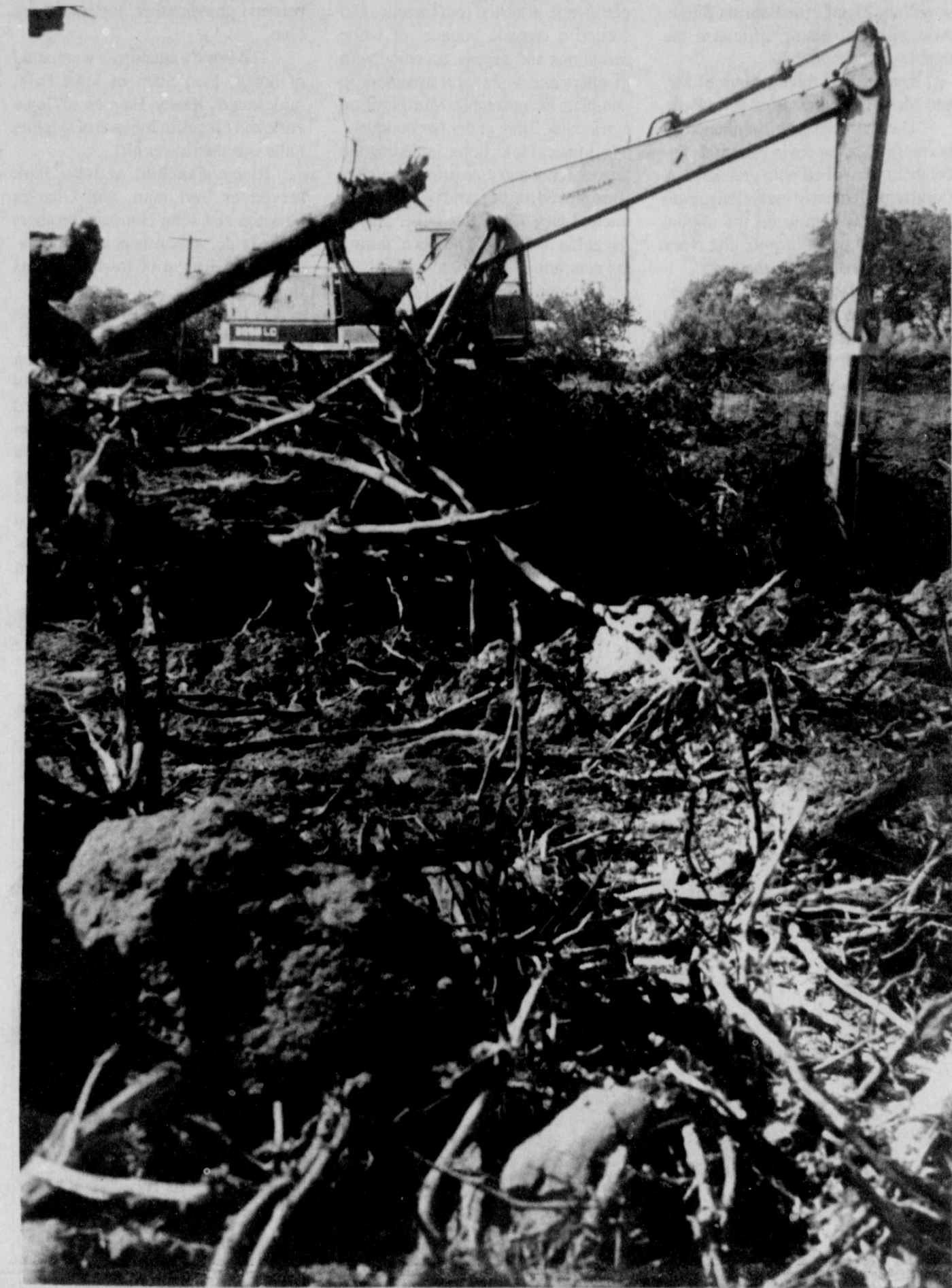
NO BURIED TREASURE - As heavy equipment began leveling the parking lot area at the new Recreational Activities Center, they discovered part of it would be directly above a deep pit of buried brush. Because of settlement over the years, the debris had to be extracted and fill soil used to level the pit before paving can be done. When the city purchased the property several years ago, it was covered almost solid with trees and brush. Workers cleared the land, and buried the debris, rather than hauling it away.
