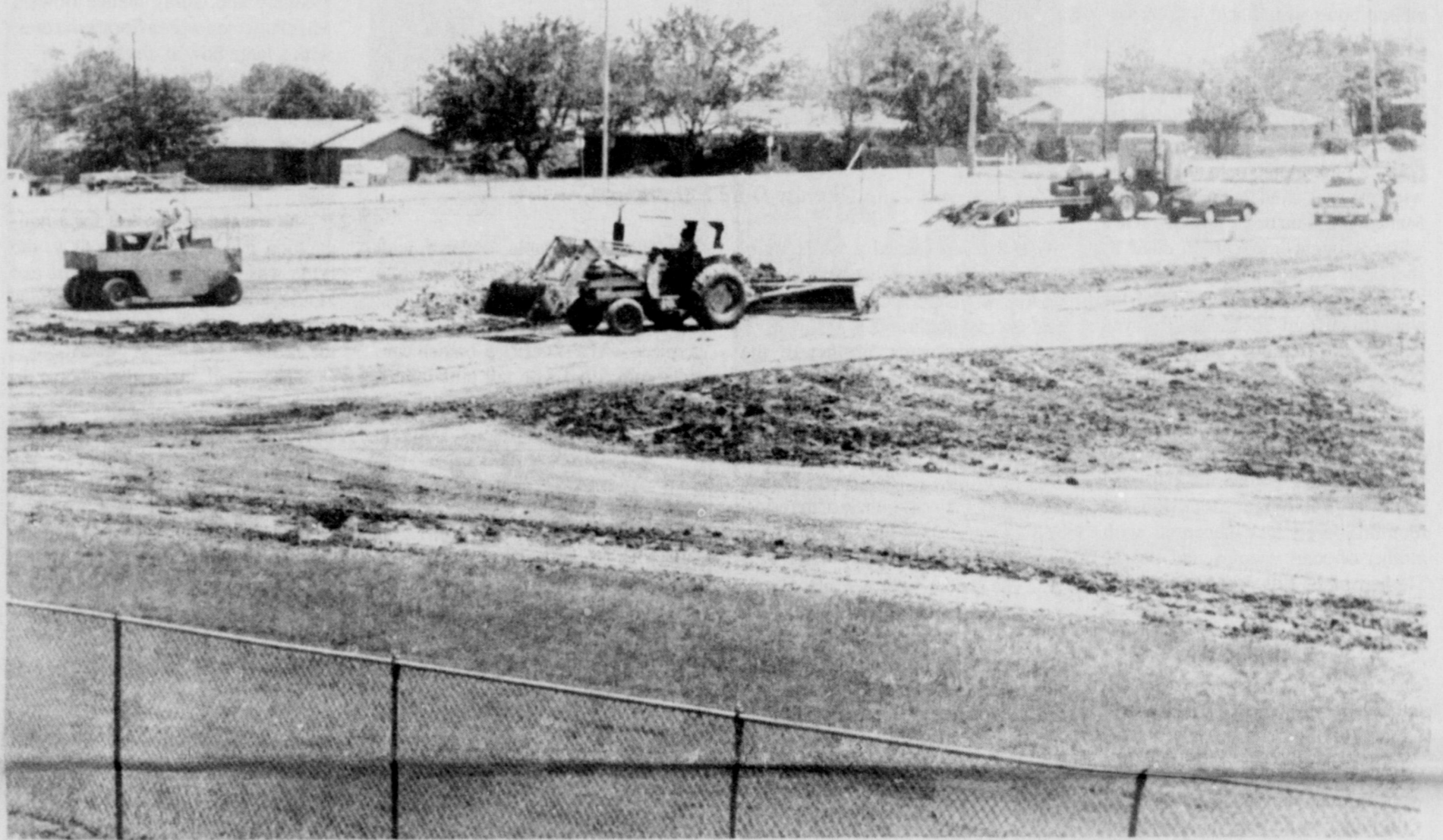
CONSTRUCTION UNDERWAY - It will not be completed before school starts, but construction is underway on a new bus maintenance facility, located south of Hawk Stadium. Trustees recently
