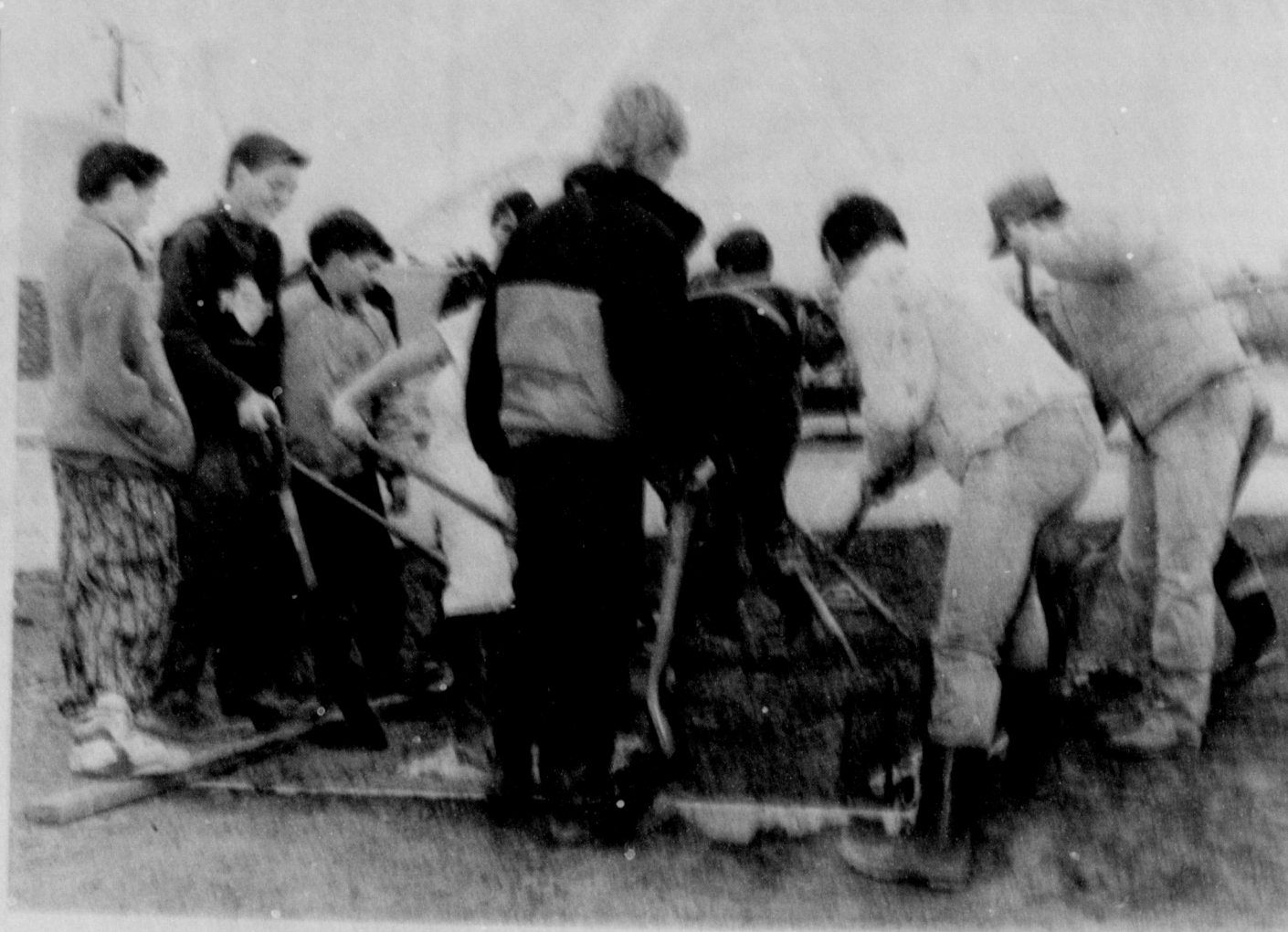
A LASTING PROJECT - Students of George Brandt last week poured the concrete foundation for a flag pole in front of Iowa Park Junior High School, in preparation for next week's open house.
