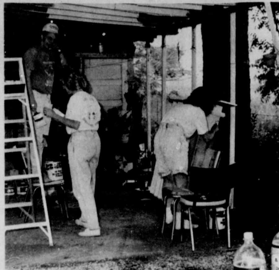
CHRISTMAS IN SPRING - Volunteers from the Iowa Park Optimist Club and Local Union 2771 made extensive improvements on a home in the 400 block of West Jefferson Saturday. The same day, here, in Burkburnett and Wichita Falls, more than 600 volunteers participated in the "Christmas in Spring" project, which is designed to make home improvements for the elderly and handicapped. Their lunches were prepared by the Iowa Park MuleSkinners.
