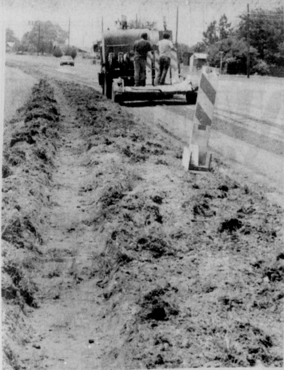
FINAL PHASE OF WEST HIGHWAY WORK STARTED ... after initial work began in January, 1990.
