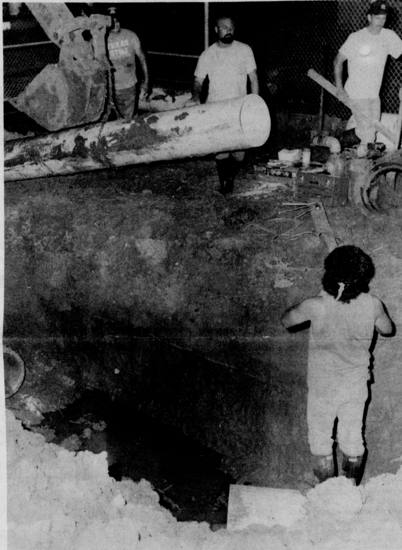
CITY WATER CREW BEGINS COMPLETION OF RAW WATER LINE TIE-IN AT PLANT ... renovation of plant became problem when transmission line from Wichita Falls had leak.
