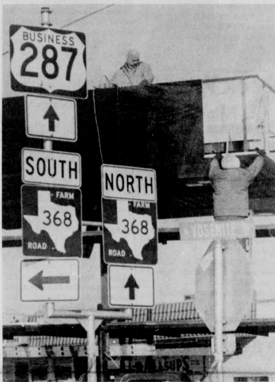
TOUGH WORKING CONDITIONS - Possibly the two most uncomfortable workers in Iowa Park Tuesday morning were the men who were replacing the metal sheeting above the gas pumps at Allsup's. The temperature was well below freezing, and the wind made it feel well below zero.
