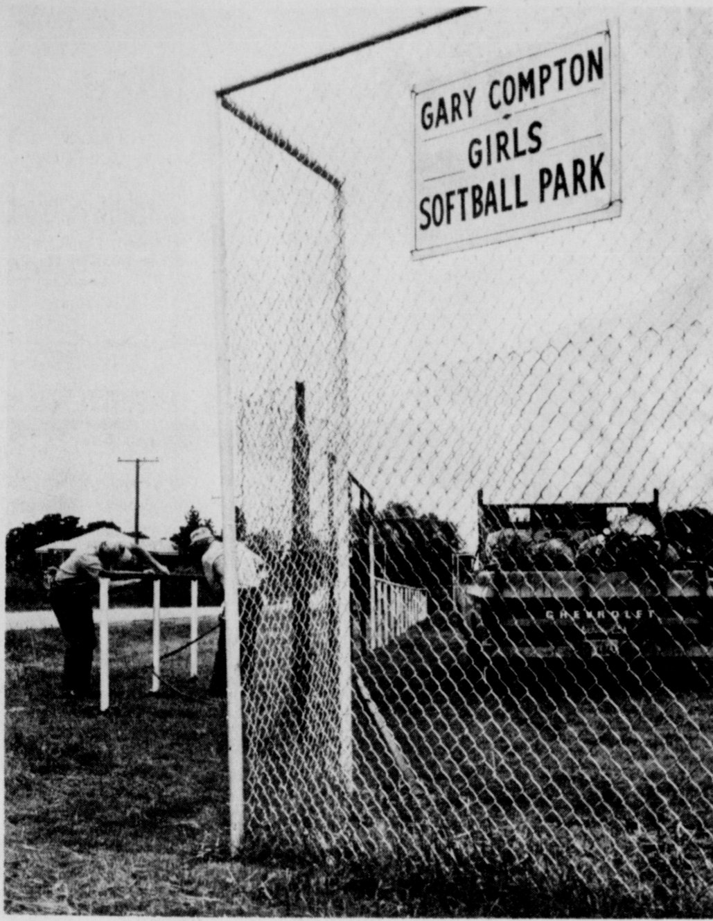
GETTING READY - Volunteer workers are frantically working to have the new fencing ready for Monday's opening of girls softball league play. A plea for additional help Saturday and Sunday has been issued for workers to complete the work. The field is located on Atlantic Street, or Bell Road.
