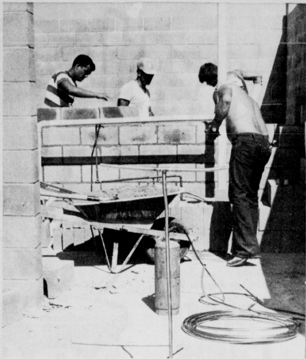
CONSTRUCTION UNDERWAY - With Monday marking the first anniversary of the Iowa Park Bicentennial Swimming Pool, construction on the bathhouse is nearing completion. The structure, which will also house an office and concession area, was not built last year due to a lack of funds. Money is still needed to pay for the building, and donations are being accepted to the "Pool Fund" at State National Bank.
