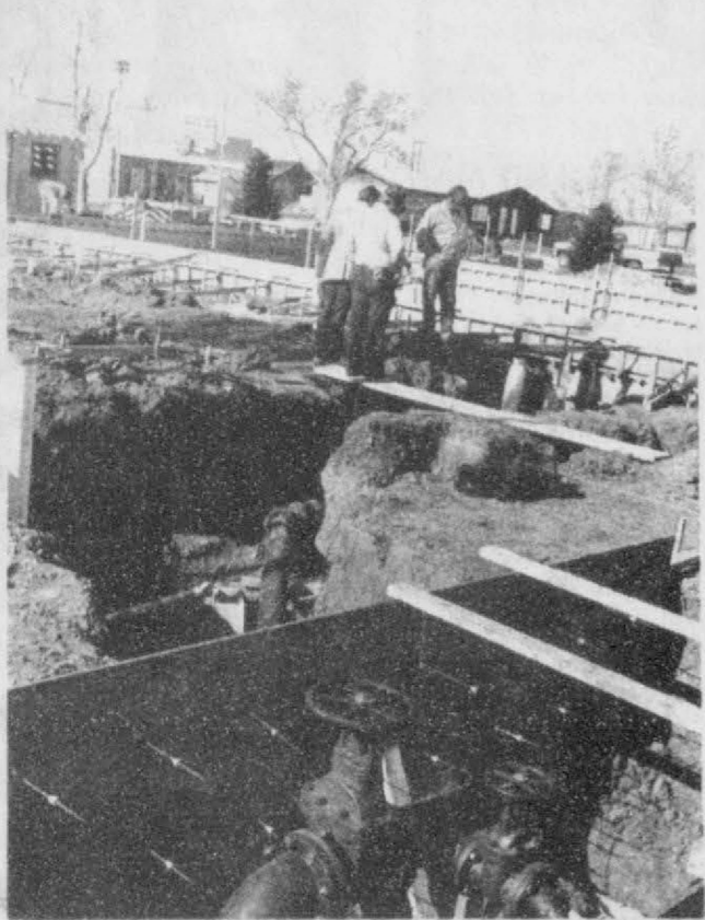
Workers have installed the water system for the new Gruver swimming pool.
