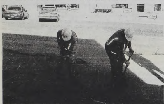
TxDOT workers repair Main Street in Quitaque after a main water line broke over the weekend.
