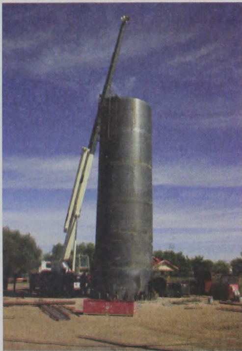
The Quitaque new water tower project is now back on track and scheduled to be completed in a few weeks according to Circle P Construction Co. spokesperson.
