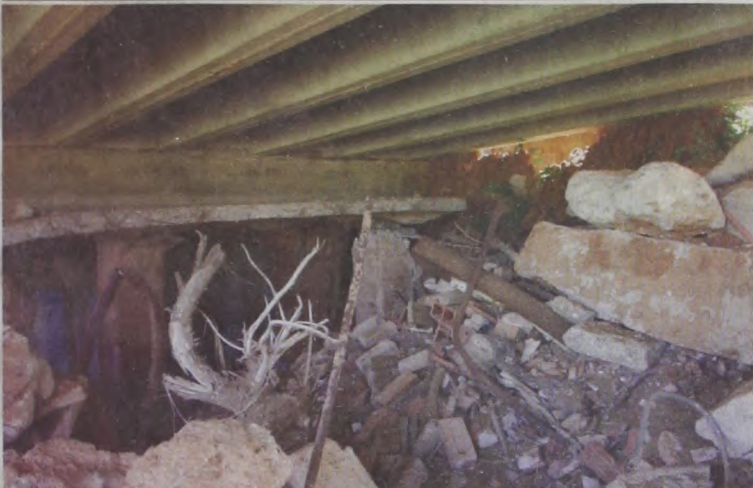
This bridge on FM 599 between Flomot & Quitaque is not even one of the eight structurally deficient bridges listed in Motley County. It passed inspection!
