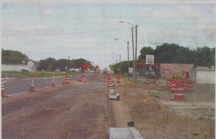
The $3,500,000.00 sidewalk renovation project continues in Quitaque. After months of construction, residents have become accustomed to detours. Sidewalk renovation projects like this have also been completed in Childress, Wellington, Clarendon, and Paducah (part of the Childress District) in the last several years. A bike/hike trail will also be installed from town to Caprock Canyons State Park along FM 1065.
