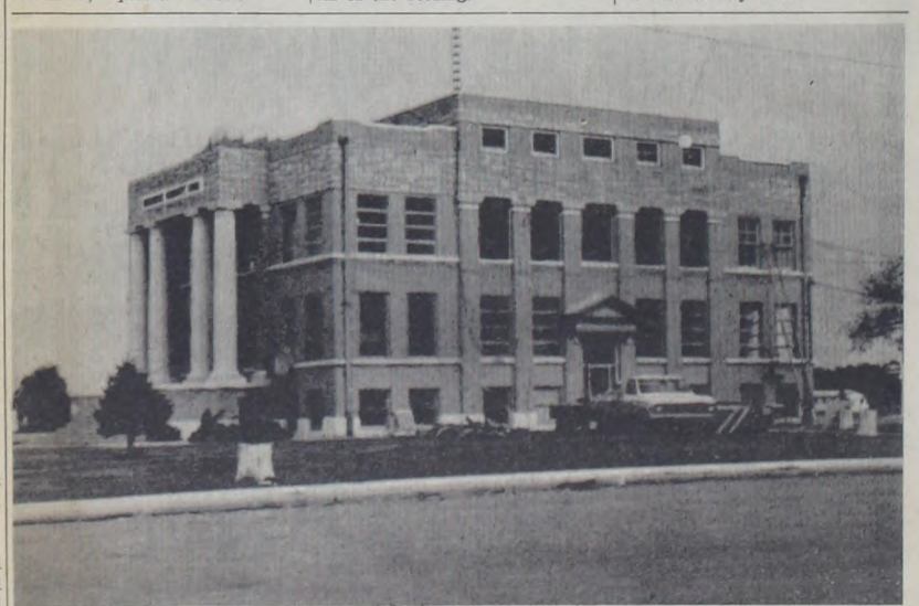
New aluminum-frame windows are being installed in the Briscoe County Courthouse. The project is being completed with money the county has received from the new revenue sharing program. (Briscoe County News Photo)
