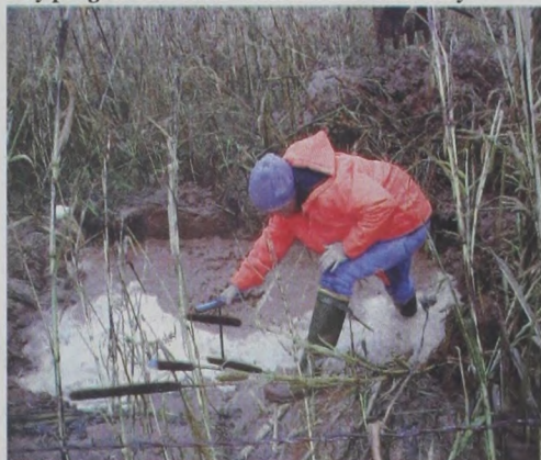
Quitaque Water Superintendent, Walter Skinner works to repair a water main break on Tuesday.
