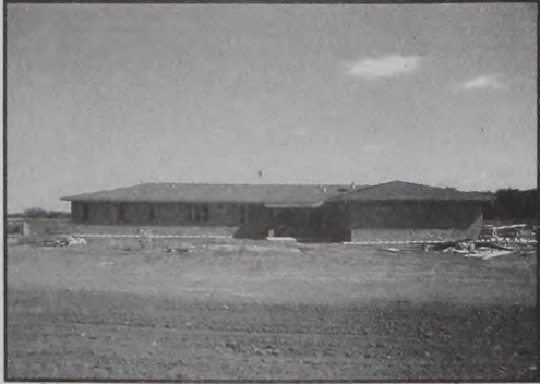
This new home currently being built just north of Quitaque is a good sign of things to come!
