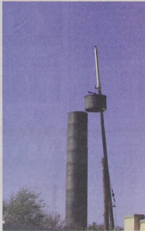
The top was placed on the new Quitaque water tower last week, now all that is left to do is sandblast & paint.
