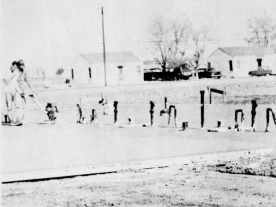
FINISHING FLOOR -- This is a picture of the Muleshoe Ranch Motel floor being finished. Machines are being used to smooth the concrete. The building site is located west on Highway 84.
