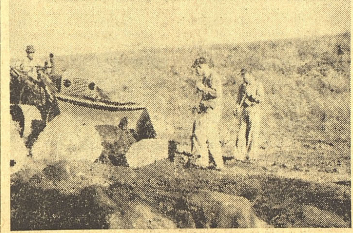
BUILDING ROADS — City workmen began building a new road around Lake Cisco Park last week. The above picture shows John Love on a bulldozer with Dero Rains, left, and Clyde Custer helping move huge stones that form borders for the new road. Motorists will no longer be allowed to drive inside the park.
