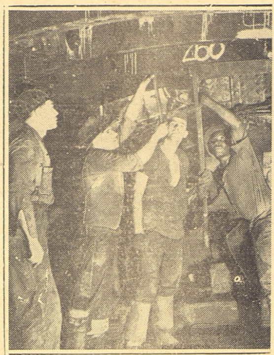
A mile and a third—7,000 feet—under the Hudson goes the newest link between New York and the mainland. Working under terrific pressure to keep back the Hudson river's water and quicksand, 8,000 men dig the opening, then line the monster hole with steel rings. Here they tighten bolts on the rings.
