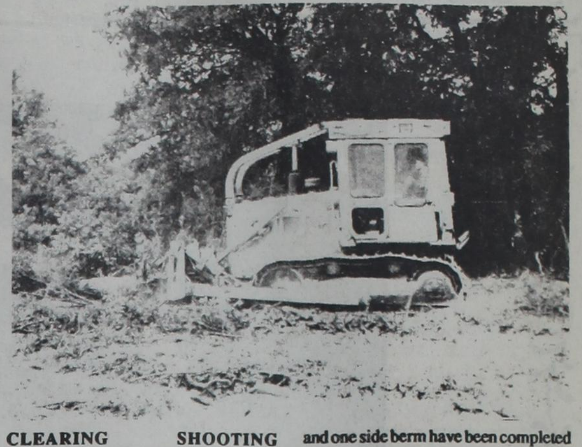
CLEARING SHOOTING RANGE —David Nichols of Nichols Dozers works at clearing the location for the rifle range at the Callahan County Shooting Range between Clyde and Baird on FM 18. To date, the backstop and one side berm have been completed Upon completion the rifle range will consist of a covered firing line 110 feet long with 20 firing stations out to a range of 100 yards.
