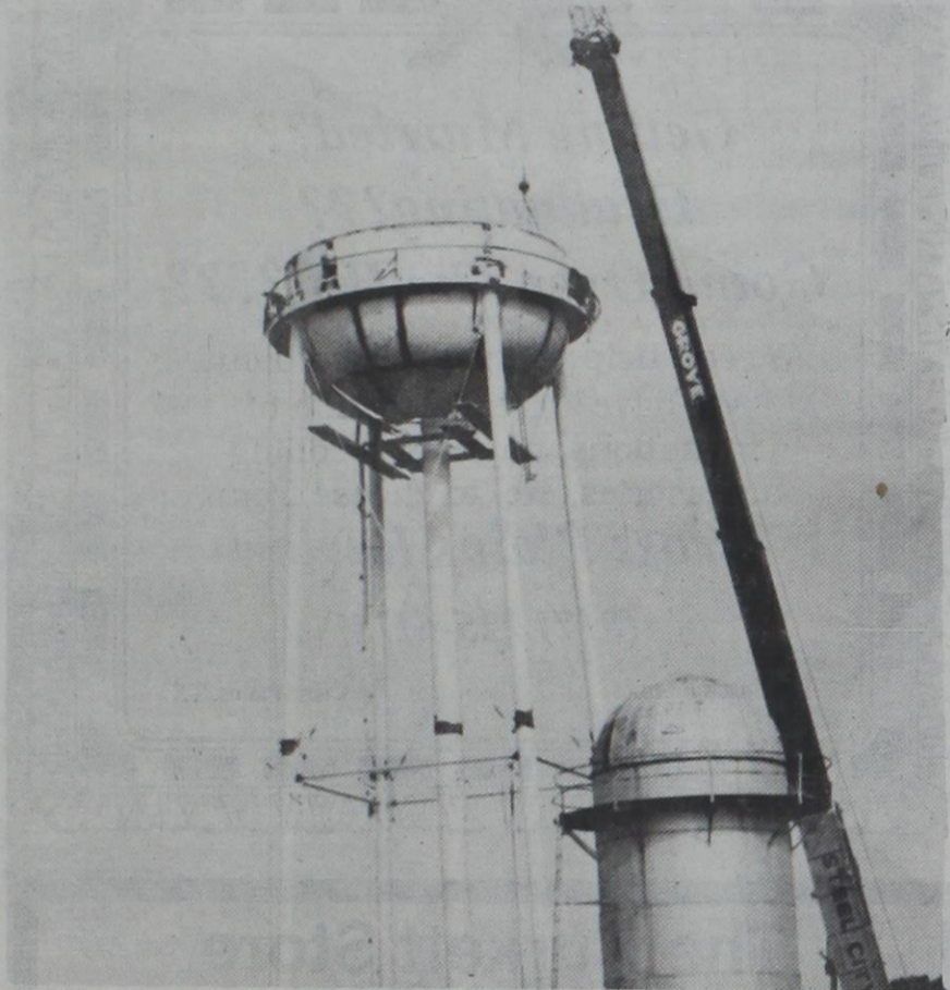
LOWER HALF OF TANK INSTALLED—A huge crane lifted the tank into position. Compare the size to
