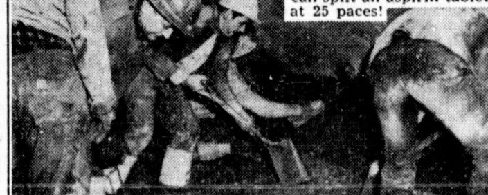
MAMMOTH MUD BATH completes ceramic tile ceiling in Lincoln Tunnel between New York and New Jersey. Tiles are first placed face down on a support 13 feet above the tunnel roadway. Reinforced concrete follows. Ceramic tile is used on tunnel walls, too, because it requires little maintenance.
