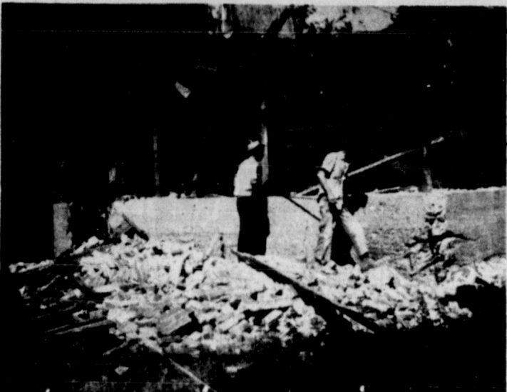
The old brick building that stood just south of the old Bartlett Motor Co. Building was being torn down the past week. The building once housed the Ice Plant. It was the last Ice making Plant in Clarendon dating from pioneer days. Pat Robertson—Staff Photo
