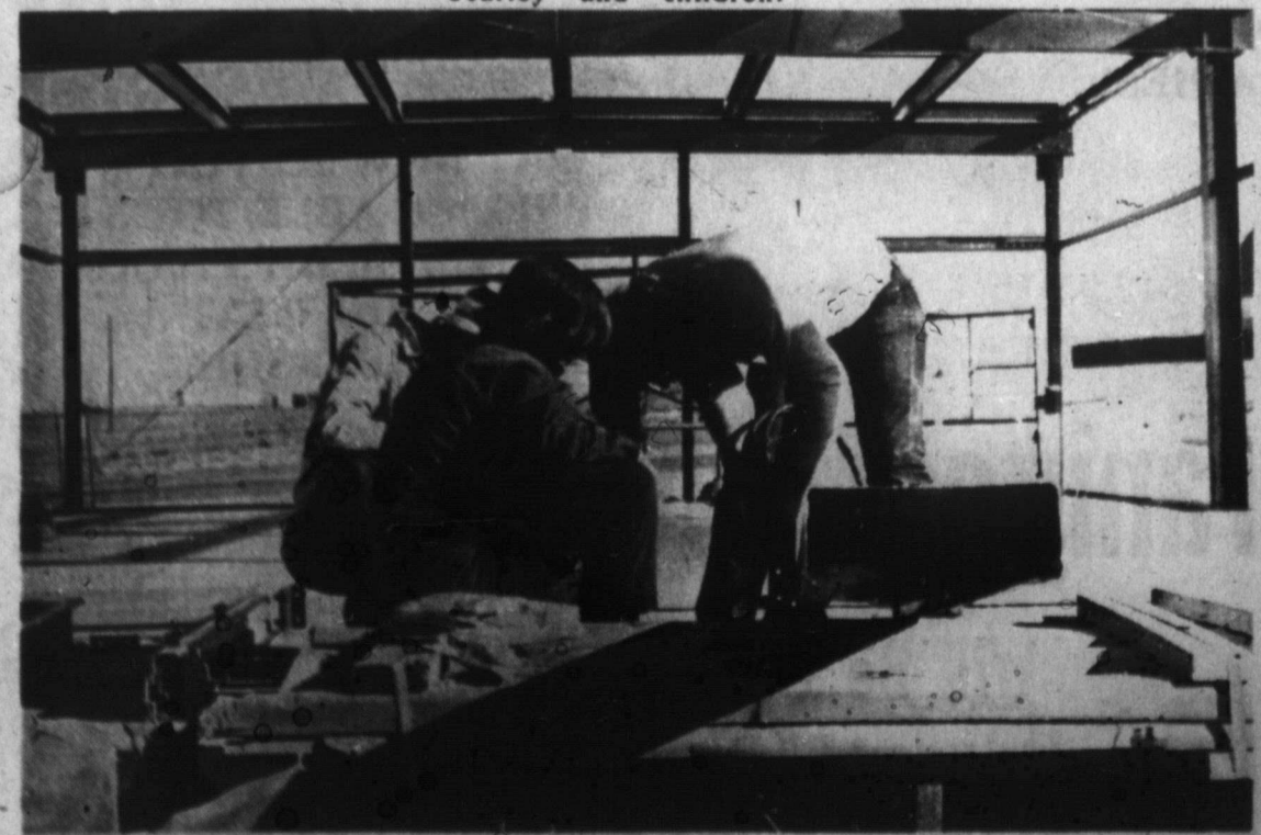
Howardwick Community Center workmen Bobby Woodrell, Ricky Brown and David Cragill said they hope to have the structural steel and sheet metal work completed by Christmas, depending on the weather. Arapaho Truck and Equipment Service of Amarillo subcontracted the job from Panhandle Steel Builders. The new facility stands next door to the Howardwick First Baptist Church, on the north side of Greenbelt Lake. Work started December 13.
