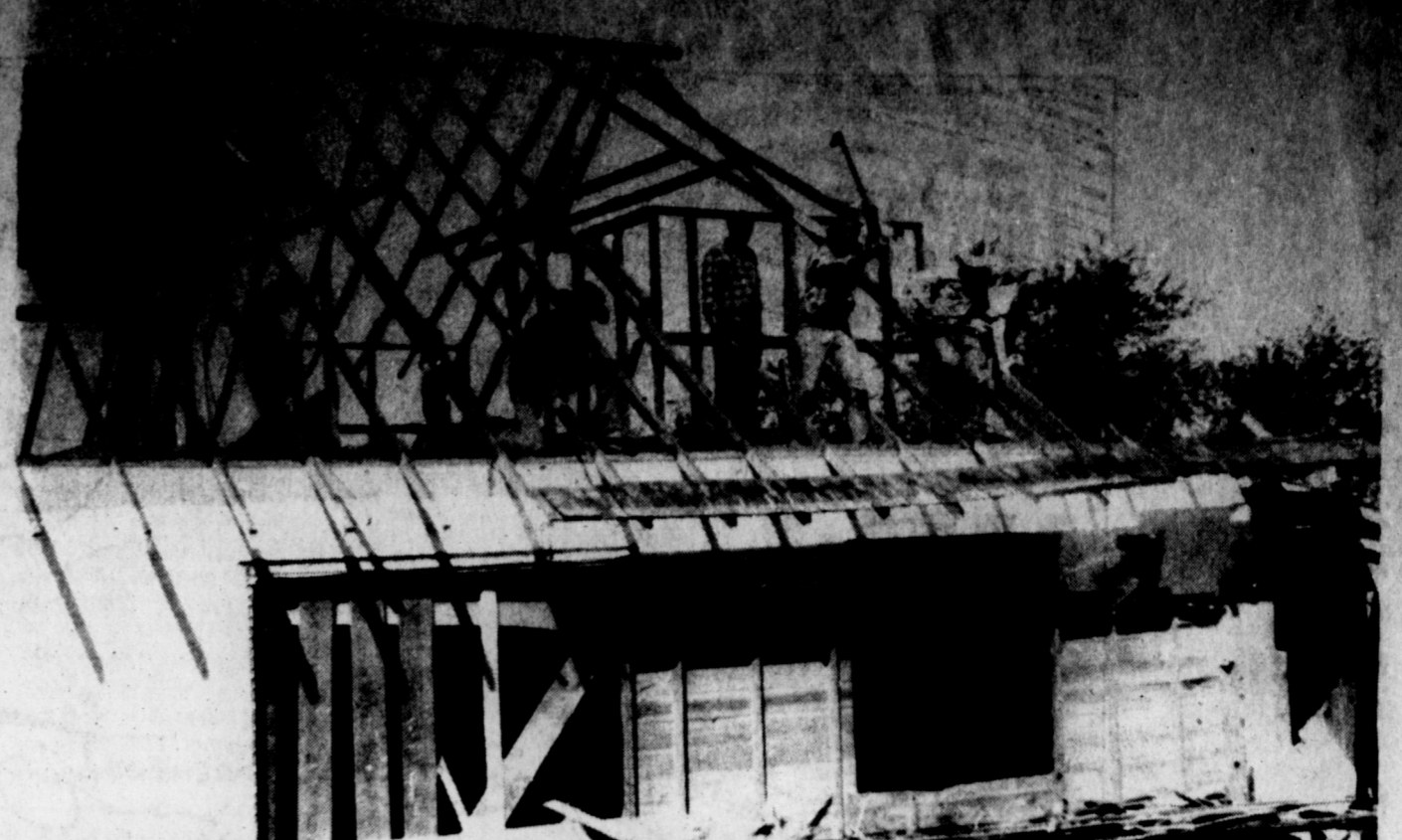
TROOP 433 Scouts, fathers and Church of Christ men completely tore down the top floor of this building, donated to the Scouts by the Church of Christ. The Scouts are building a Scout house on property donated by Claude Thomas. Tommie Saye Troop 433 Scoutmaster would greatly appreciate any help, either labor, material or funds. Any money donated for this project will 100% stay in Clarendon to be used toward building this Scout house for Clarendon Scouts.
