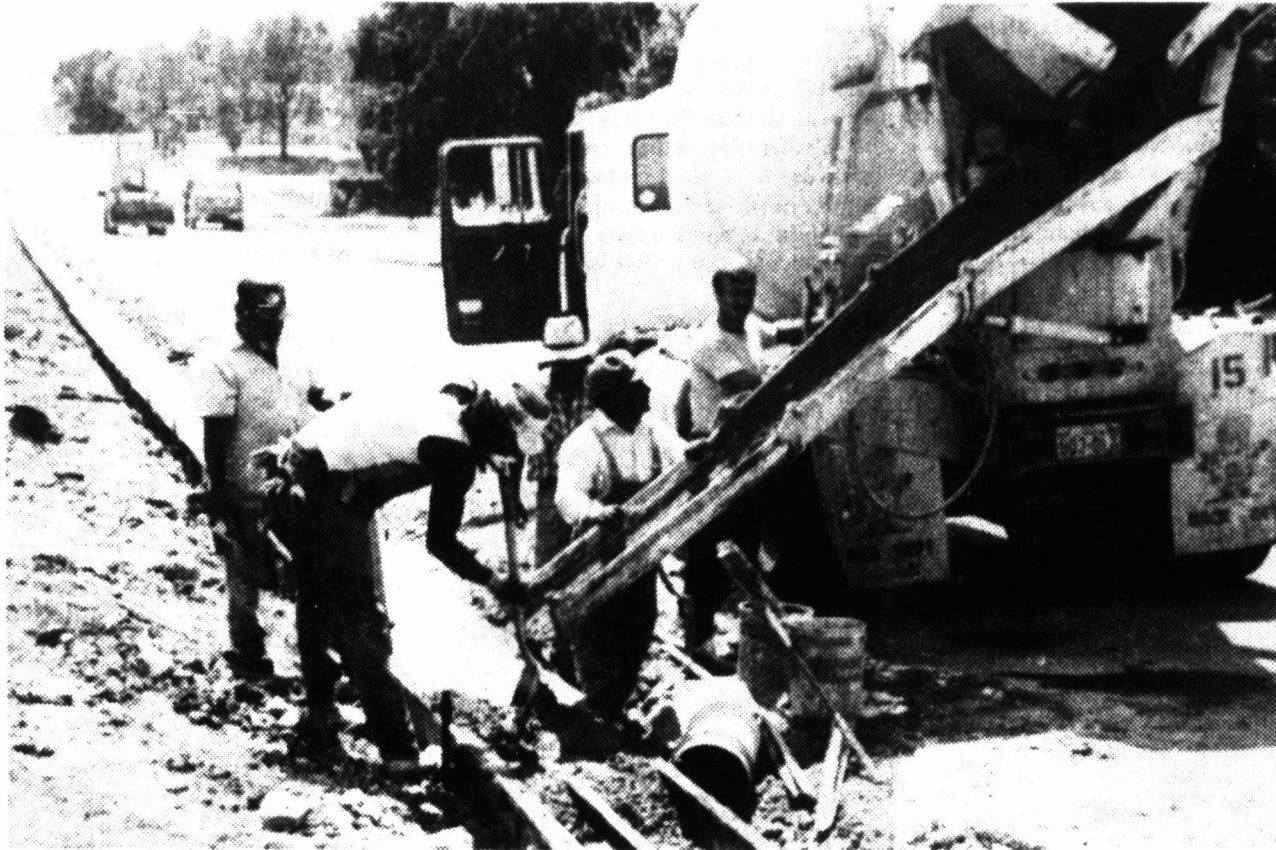
CURB AND GUTTER WORK. Contractors have installed curbing and gutter along both sides of Bugbee for about two blocks south of Hwy 287.
