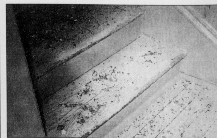
The stairway leading to the attic is covered with guano, and the stench at this point is very prominent. In the attic itself, piles of the feces are as high as ten inches in some places.
