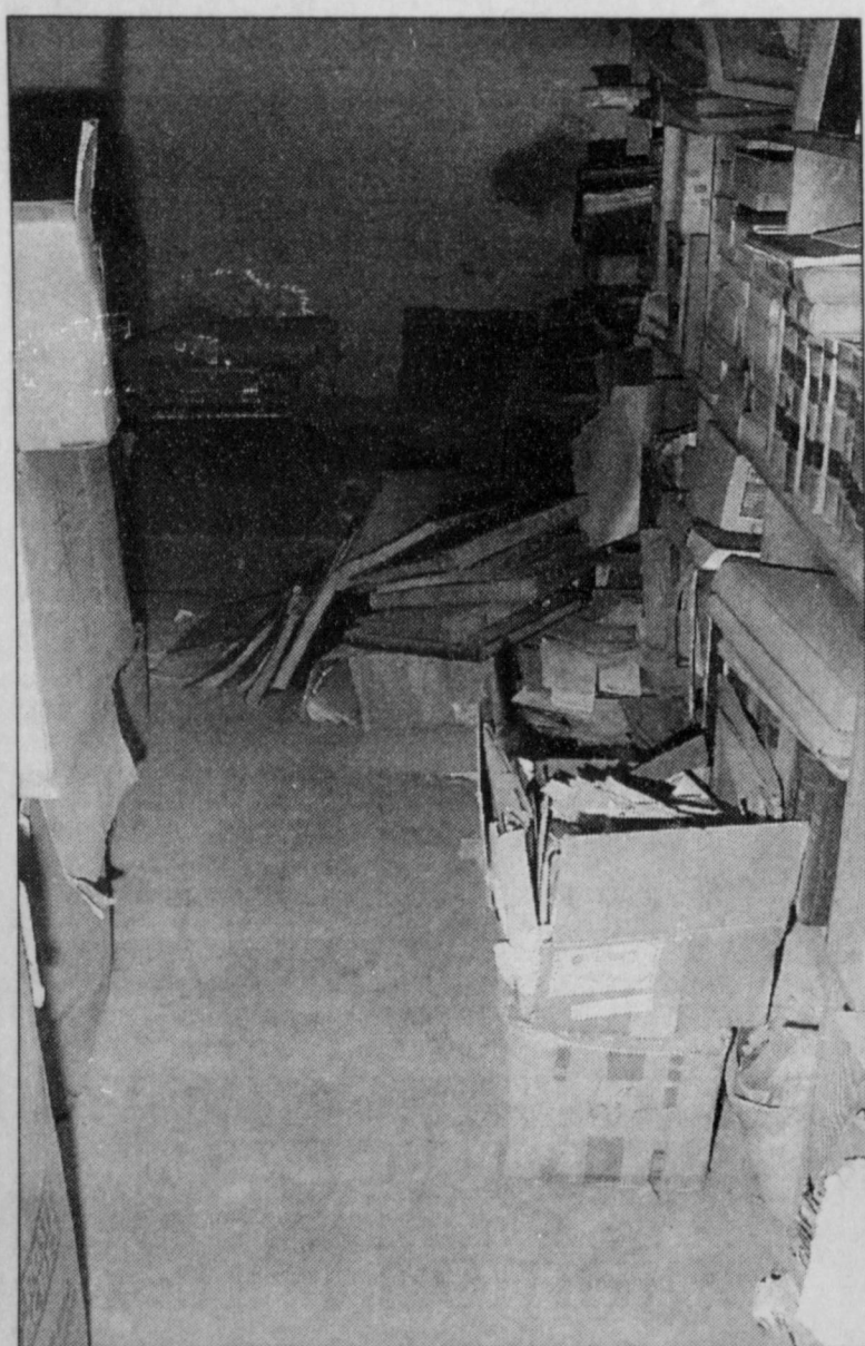
Many of the county's old records are stored just like this — piled around on the basement floor. Sand covers the floor and the records in this room as it falls from the mortar joints of the walls, which are being damaged by moisture. Drainage around the building must be corrected to prevent further damage to the basement walls.
