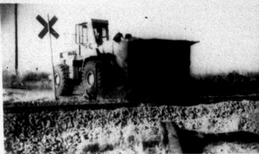
AFTER RENOVATING THE FOUNDATION beneath the track, Burlington Northern crews are reworking crossings to make them safer and smoother. The first step is to build up the crossing so that the road bed is level with the rail head for twenty feet on either side of the track. In the picture above loader operator Charles D. Sherman builds up the new crossing with fill dirt.
