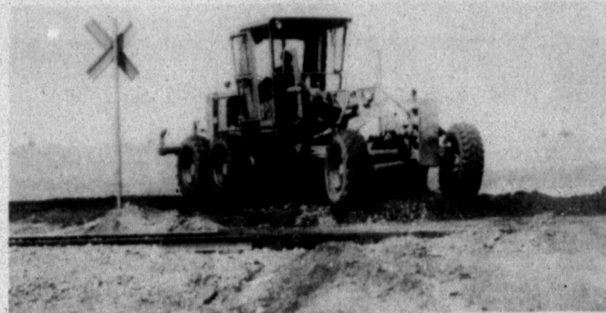
THE FINAL STEP in upgrading the crossings is smoothing and packing the surface. The roadways are surfaced with tailings from the undercutting machine, a mixture of gravel and fines that makes a good road surface. The taller crossings raise the driver's visibility above the weeds, give better drainage and make it easier for vehicles to get on across the tracks. Charles Gullede of Childress is in charge of the renovation. Like all the Burlington workers who visited with The Clarendon News Gullede is concerned about crossing accidents in the area.
