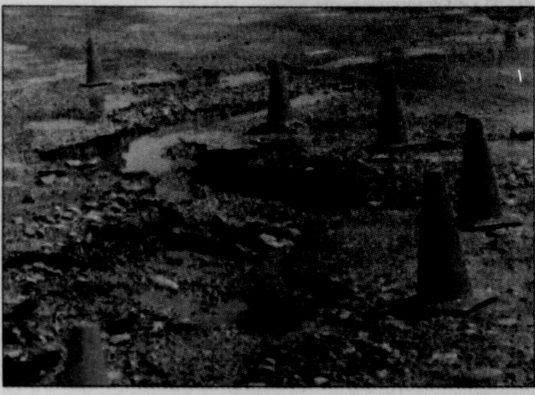
Parks Street took a heavy toll when 2.5 inches of rain hit the city early Sunday morning. Local officials hope to prevent future damage such as this by implementing a $2.5 million plan for street and drainage improvements.
