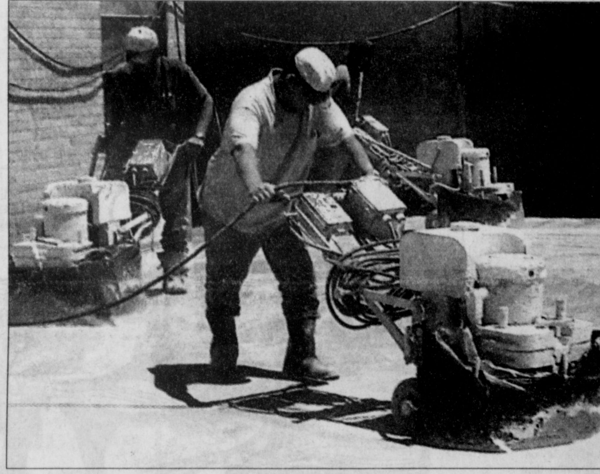
Jerry Sawyer, Mike Henley, and Benny Martinez of Zanchettin Brothers Tile & Terrazzo in Amarillo polish what will become the new main corridor of Hedley High School.
