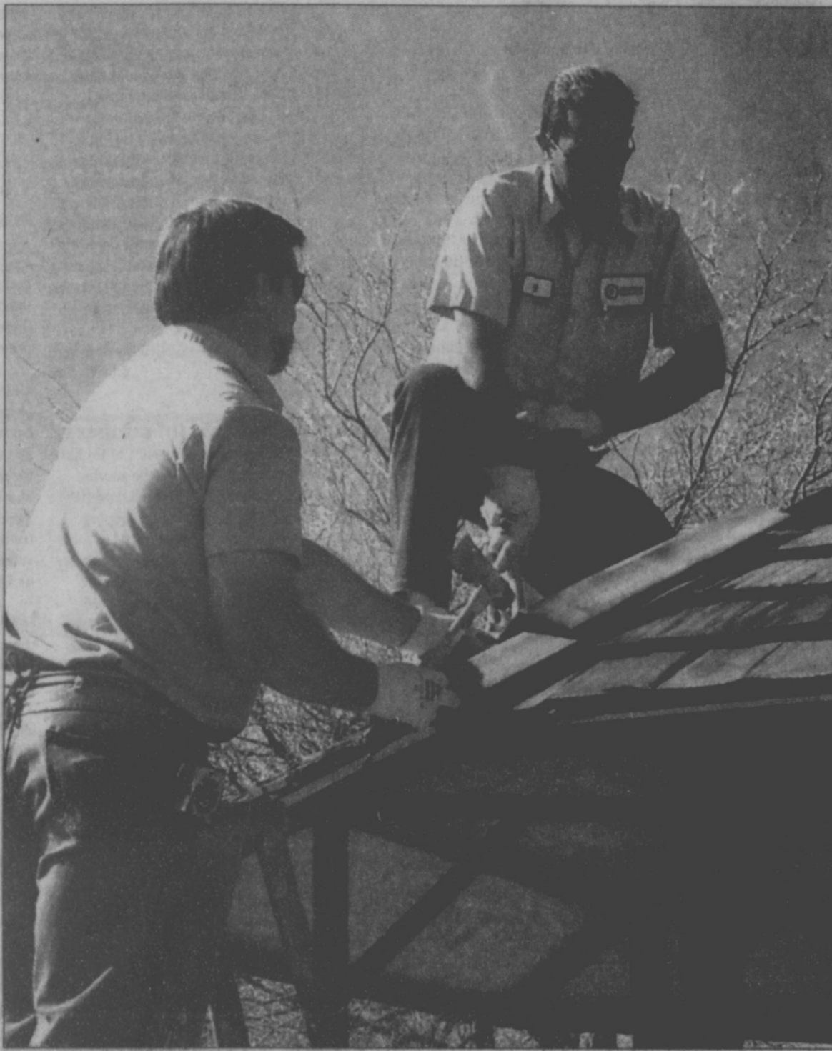
Top it off Greenbelt Water Authority employees Jeff Topper and Roy Monroe put the finishing touches on a gazebo that has been built at Sandy Beach. Several improvements have been made at the beach and at Kincaid Park over the last couple of years.
