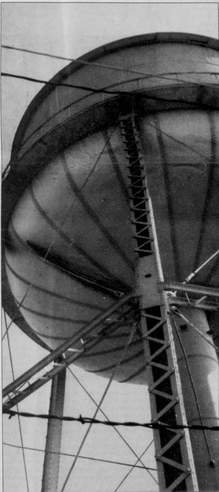
Rust runs down the bottom of the city's west water tower. ENTERPRISE PHOTO / ROGER ESTLACK
