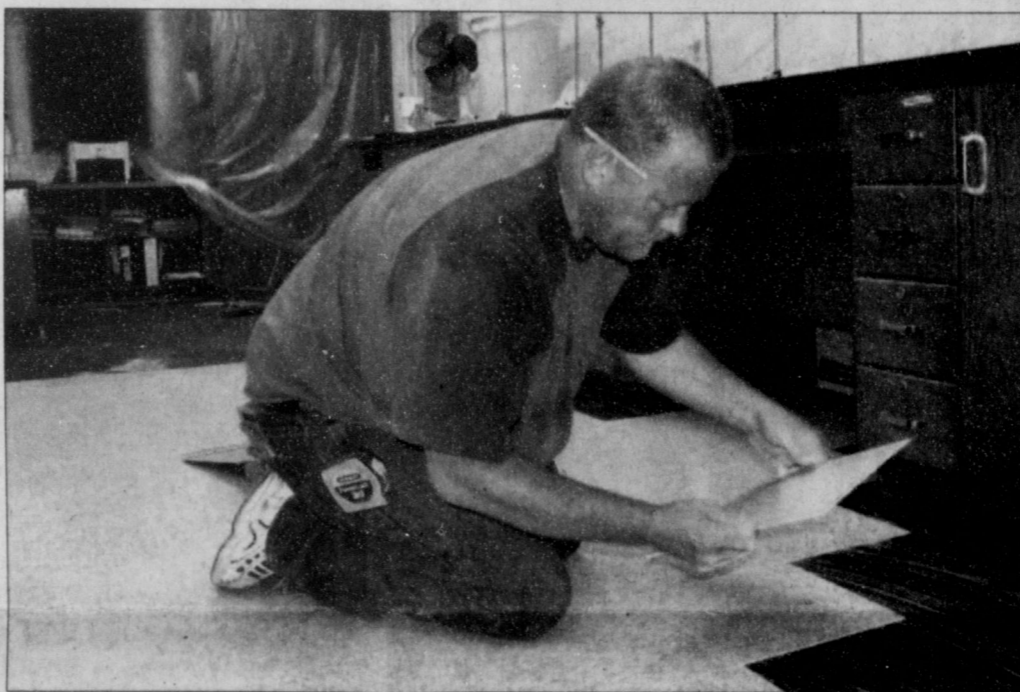
Brandon Curry paints an administrative office at Clarendon High School Monday (top) while Dayton Lovelady lays tile in the chemistry lab as part of the summer renovations taking place at the school.
