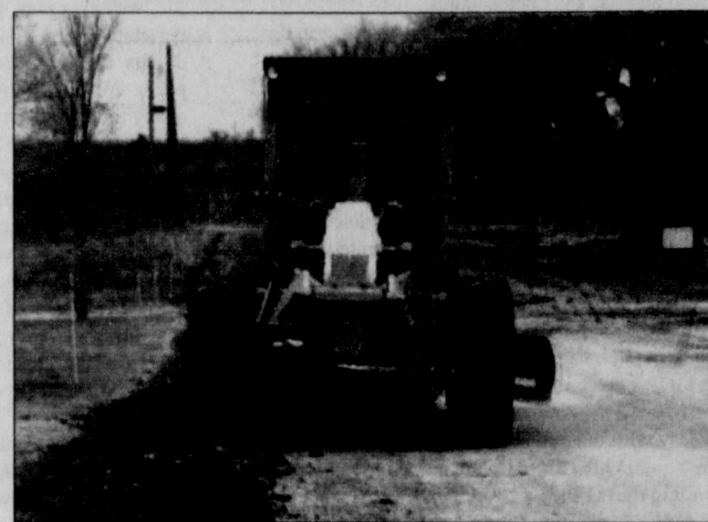
City crews began ripping up Collinson Street this week in preparation of this year's paving project, which is expected to pave and curb approximately 50 city blocks.
