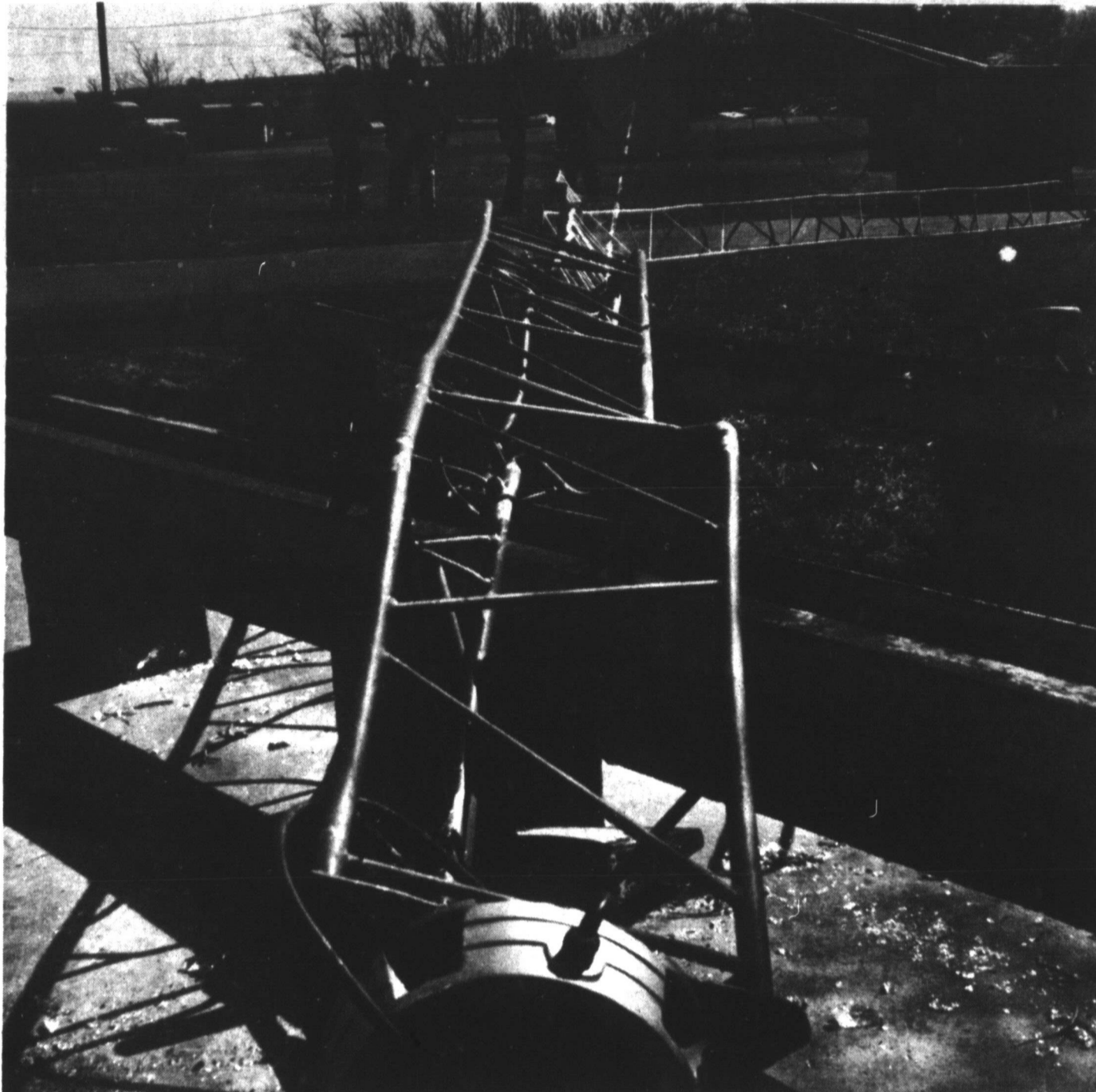
TEXAS HIGHWAY DEPARTMENT workmen began cleaning up the debris left of their 160-foot radio communications tower which toppled to the ground about 1:30 p.m. Friday. The tower kept the Clarendon office in communication with other highway department units including those in Childress and Amarillo and was also used in communicating with work crews maintaining roads in the Donley County area.
