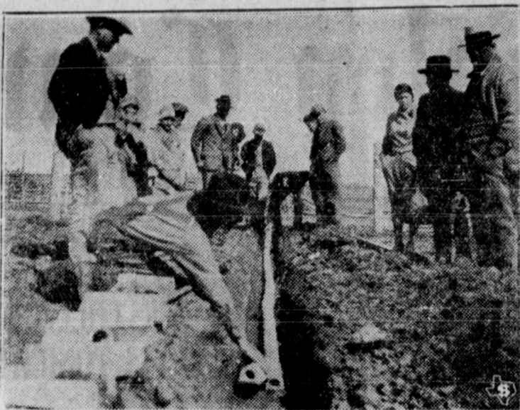
Here is shown a sub-irrigation installation in Grayson county, Texas, by B. F. Gray on the Hart farm. Sub-irrigating gardens using lath tile costing about one cent a foot is one of the big developments in gardening in Texas. The move is so strong this year that many are making cheap concrete tiles at home for the purpose.
