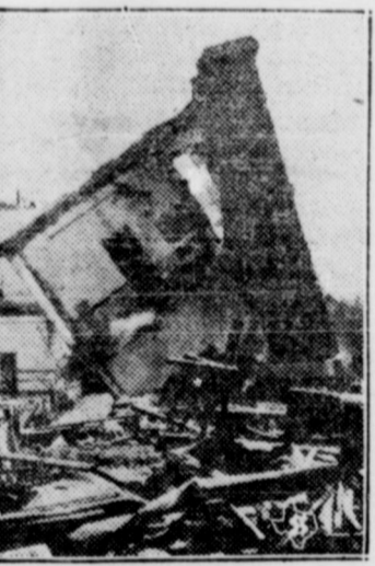
This section of the old federal building at Tyler resisted two shots of dynamite and two pulls of a donkey engine before it finally fell. The building is being demolished to make way for a new $300,000.00 structure.
