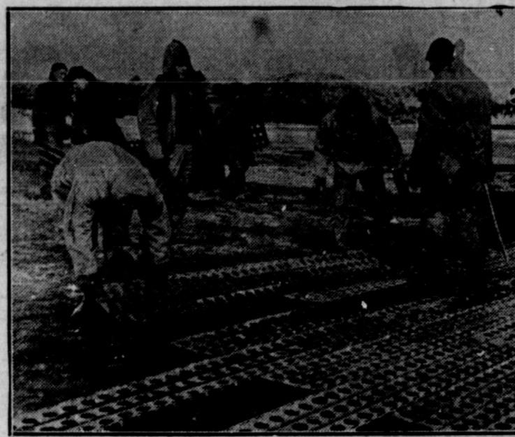
Bureau of Public Relations, U. S. War Department AVIATION ENGINEERS IN THE ARCTIC —A vital link in the chain of air bases built by U. S. Aviation Engineers is this landing field somewhere in the Aleutians. The field having been cleared, graded and rolled, portable steel landing plank is laid to complete the intricate system of runway and taxiways from which our aircraft will carry the war to the enemy.
