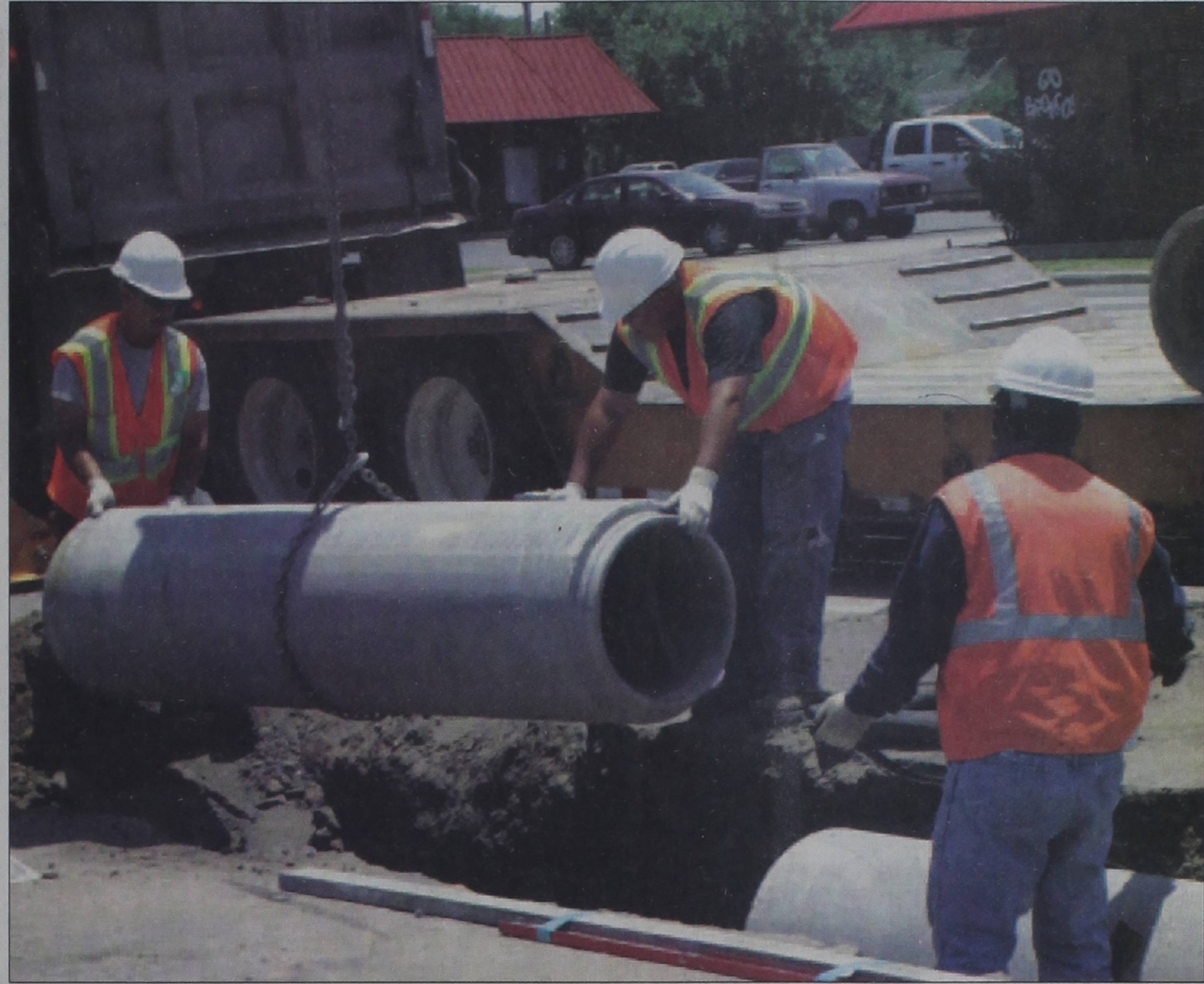
Workers with J. Lee Milligan lower concrete drainage pipe into place in front of Lowe's Family Center Tuesday afternoon as part of $1.4 million project that will resurface US 287 through Clarendon and improve drainage in trouble areas. ENTERPRISE PHOTO / ROGER ESTLACK
