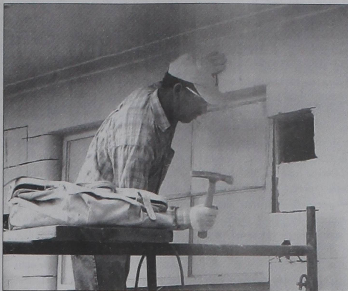
Samuel Gomez works to take out an unused window as part of renovations to the Bronco field house at Clarendon ISD.
