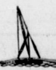
Cranes lifted each new section of pipe to a position on the barges where it could be welded to the section already laid.
