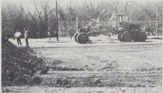
SURFACE PREPARATION began this week on the new tennis courts in the Muenster City Park, being constructed by the Muenster Jaycees. Janie Hartman Photo
