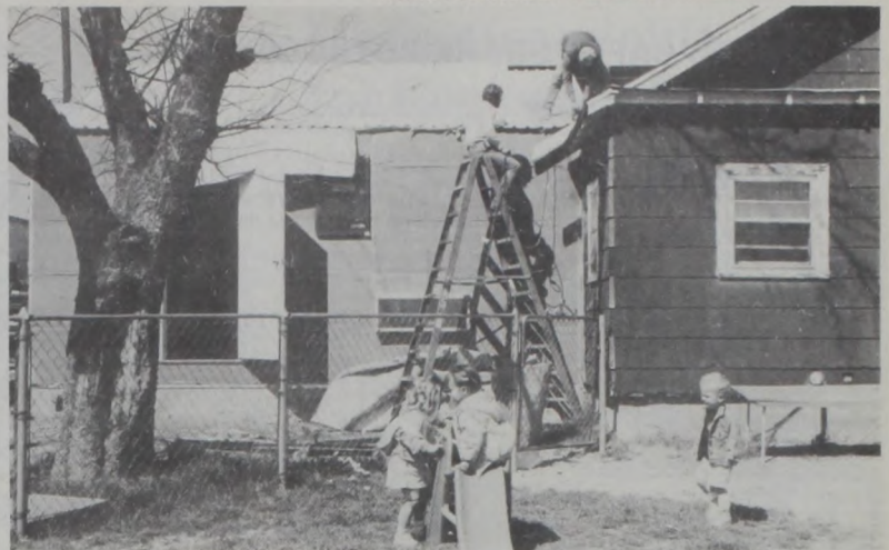
CONSTRUCTION CONTINUES at the Tender Loving Care Day Care Center. The addition will enable owner/director, Wanda Flusche, to enroll 22 more children, which will enable working mothers to have a place to leave their children. The space will also improve the overall operation of the day care. The new room will primarily be used for a large play room with a classroom set up at one end for three year olds. All the children, ages 2-5 years, will take naps in this room, which leaves the rooms in the existing building free to set up for 4 and 5-year-old classroom, 2-year-old classroom, and two separate infant rooms. Pictured are Shawn and David Flusche Jr. of Structures, Inc. in Muenster.
