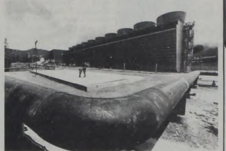
Subsurface steam developed by Aminoil USA, Inc. is spinning the turbine of the world's largest geothermal steam-powered electric generating plant.
