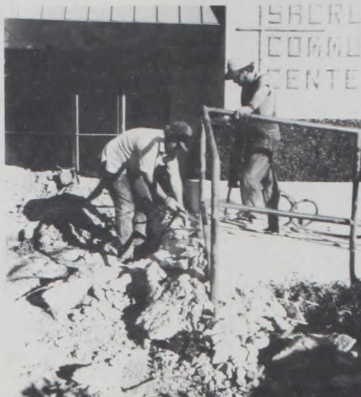
Lynn Huchton, (left), and Ernie Martin tear up the concrete steps and outside entry of the Sacred Heart Community Center. The area will be completely rebuilt because it has sunk and water has been seeping into the Community Center from under the door.
