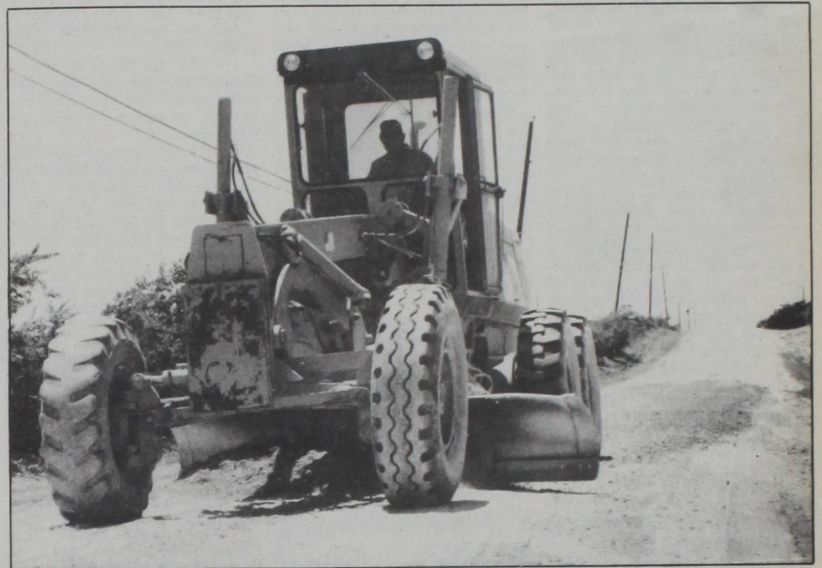
DOUG MARTIN drives a Precinct 4 road grader, preparing the base of County Road 428 for paving. Janie Hartman Photo
