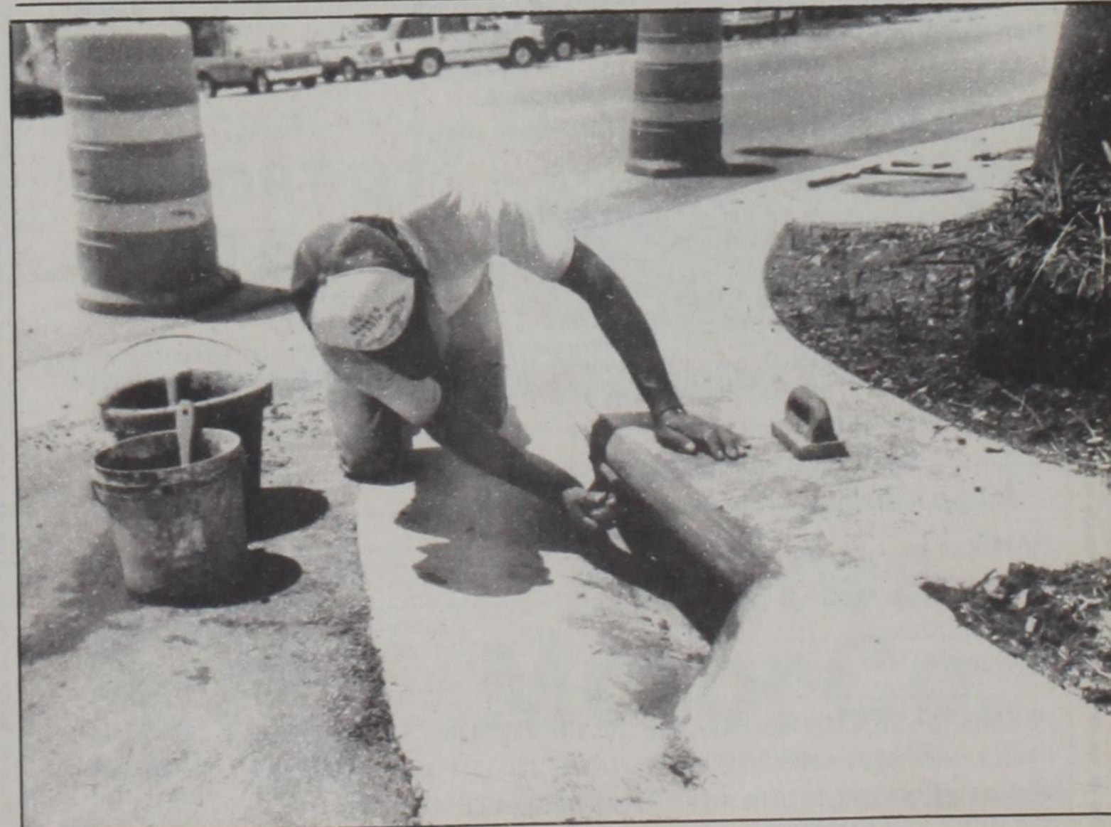
BENNY LOERA, an employee of Russell Cowan Construction Co., puts the final touches on a new corner drain along Highway 82. Construction began April 2 and was finally completed this week.
