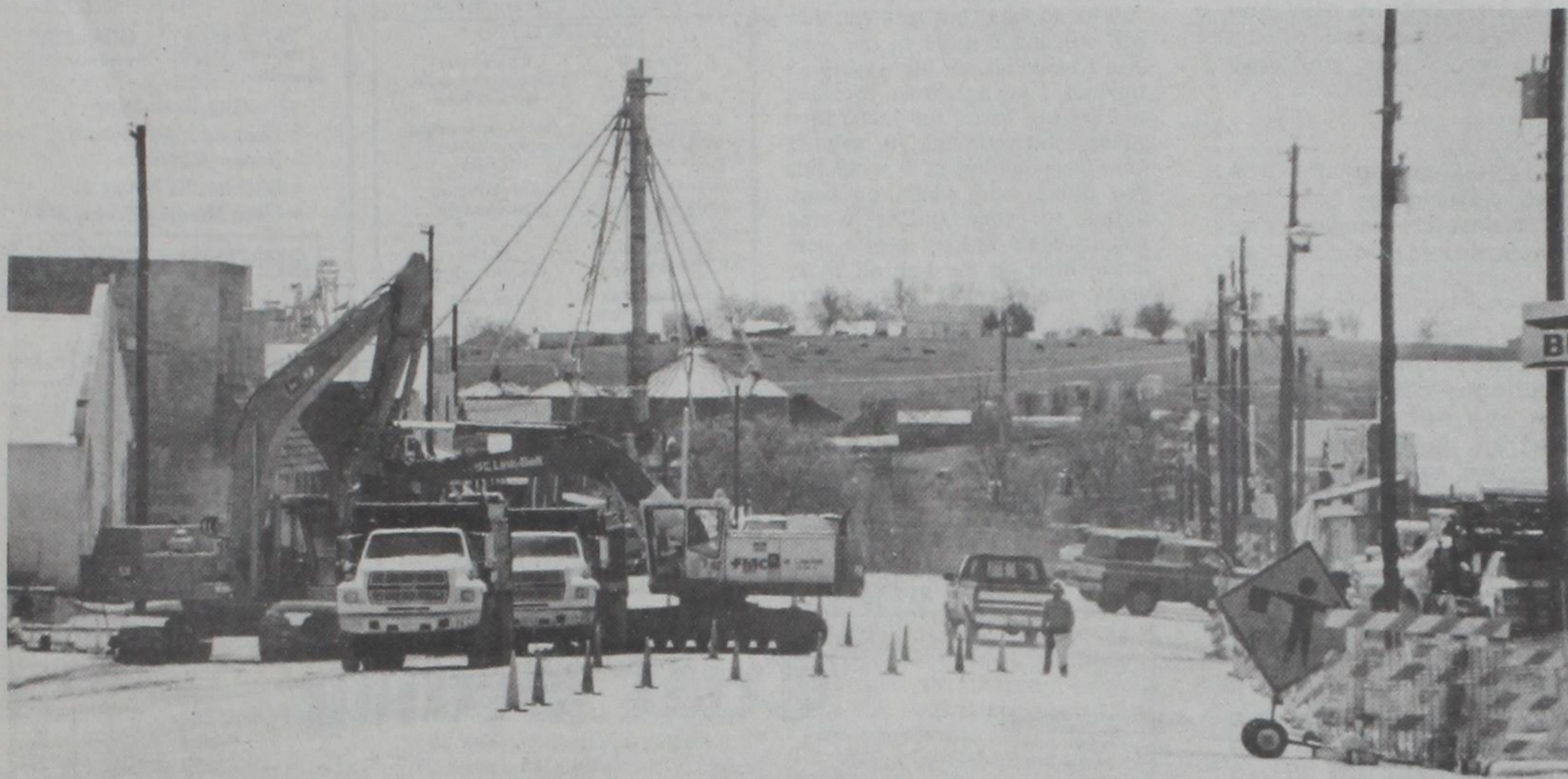
WORK CONTINUES full force on storm drain installation on Main Street this week. Dunnick Bros. Construction placed the underground pipe in the once-Main Street "dip" to improve street drainage. Traffic was re-
