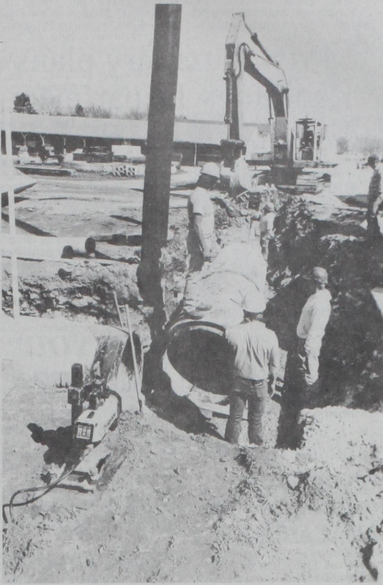
DUNNICK BROS. CONSTRUCTION started work in high gear this week after storm drain installation has been delayed for months because of the weather. Rain water control pipes are being placed on Main Street with Second and Fourth Streets drainage meeting at Third Street. An underground pipe will replace the dip on Main Street as runoff water will be channeled under the street for drainage. The job should be completed in 120 working days.
