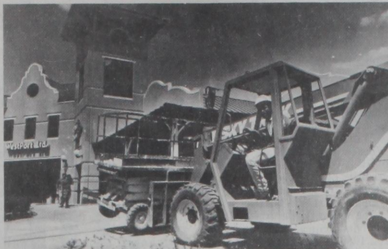
DUDE GREWING is one of many area residents who landed a job building the Gainesville Factory Shops. The center expects to bring 1,100 new jobs to this area. Dave Fette Photo
